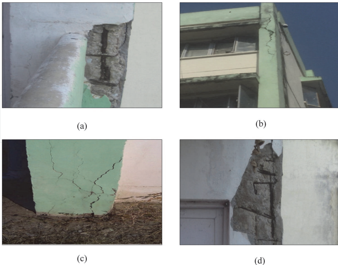
Figure 3. Damage detection (a) spalling of concrete, (b) vertical cracks on column surface, (c) cracks in the bottom of column, (d) corrosion in steel.
