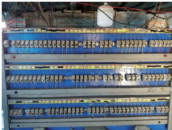
Figure 6. A miniature circuit breaker board of a neighbourhood diesel generator (Source: Author).
