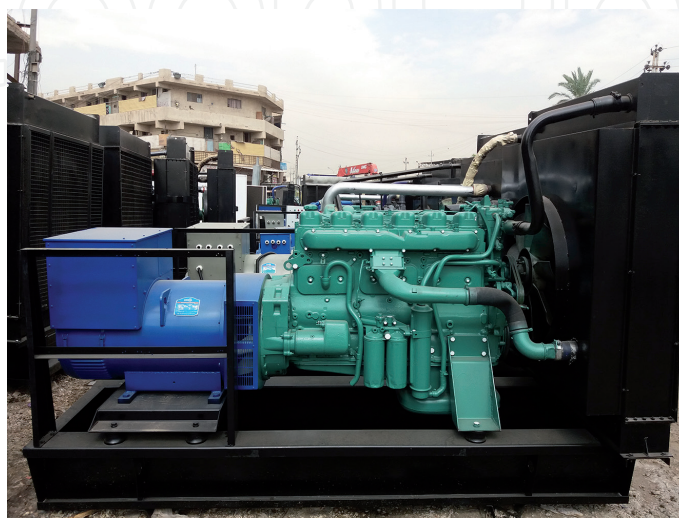
Figure 2. Locally assembled neighbourhood generator (Source: Author).
