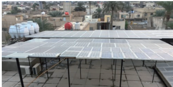
Figure 18. A rooftop array of solar panels in Baghdad (Source: Dr. Jaafar Ali Kadhum Al-Anbari).
