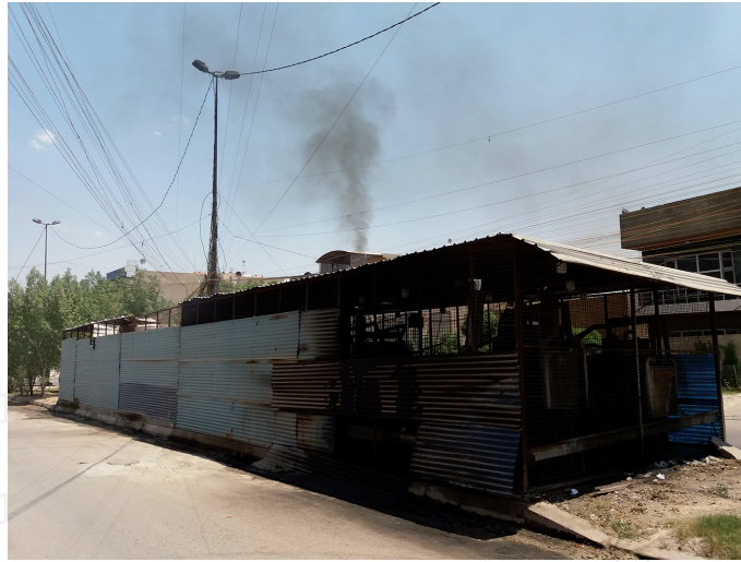
Figure 4. Neighbourhood diesel generator installed on a mid-road pavement in Baghdad (Source: Author).
