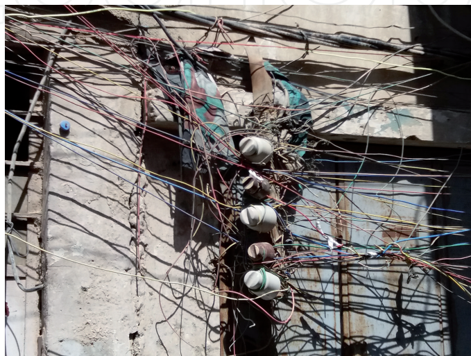
Figure 7. Informal distribution circuits using redundant utility support insulators (Source: Author).
