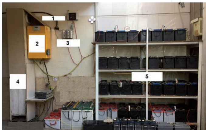
Figure 19. Detailed illustration of a 10 kW experimental rooftop off-grid solar system in Baghdad (Source: Dr. Jaafar Ali Kadhum Al-Anbari).
