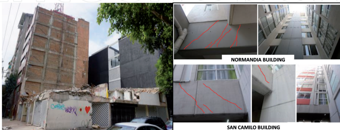
Figure 1. (a) left: Collapse of a building with discontinuities in elevation; (b) right: Diagonal cracks in the girders of the transfer floor in two buildings supporting six and seven stories, respectively.
