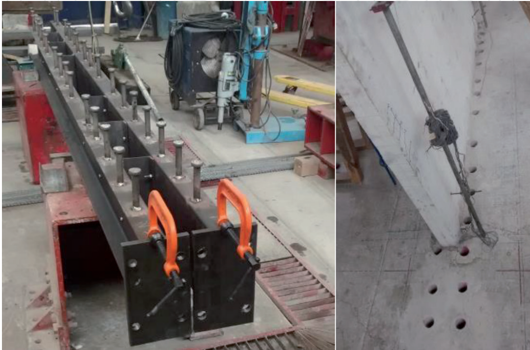
Figure 17. C-shaped steel channel with stud shear connectors (left), drills in the concrete slab.
