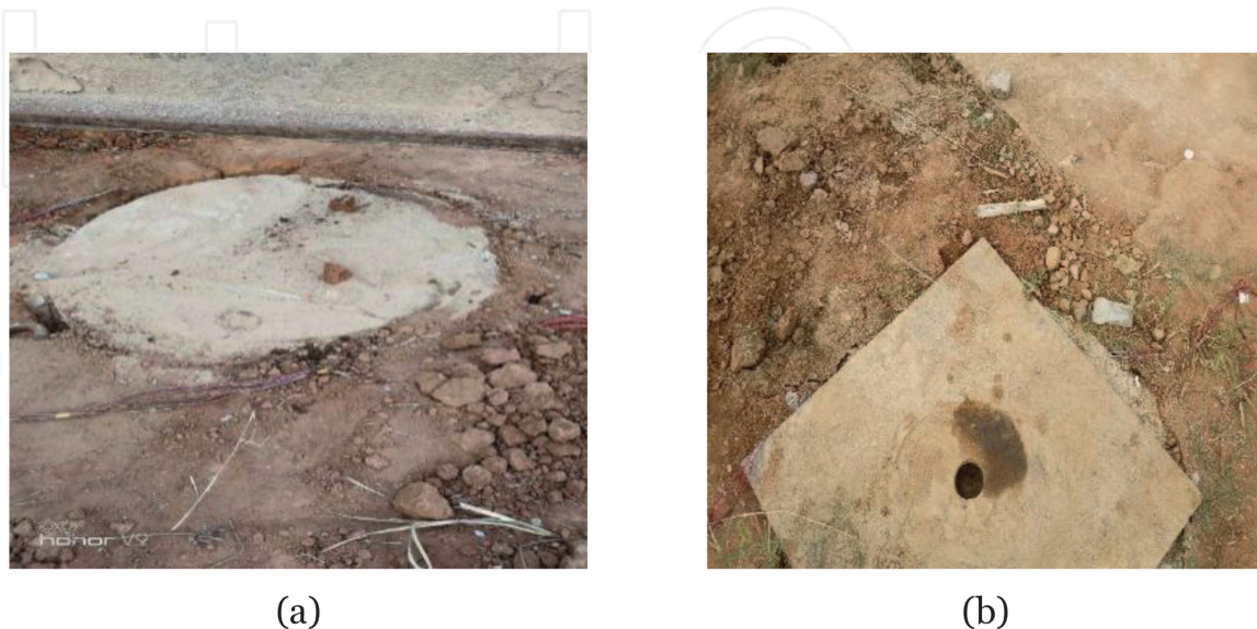
Figure 16. Failure modes of concrete piers. (a) Soil around the pier when the precast pier foundation of recycled compound concrete was destroyed, (b) soil around the piers when the foundation of the cast-in-place ordinary concrete was destroyed.
