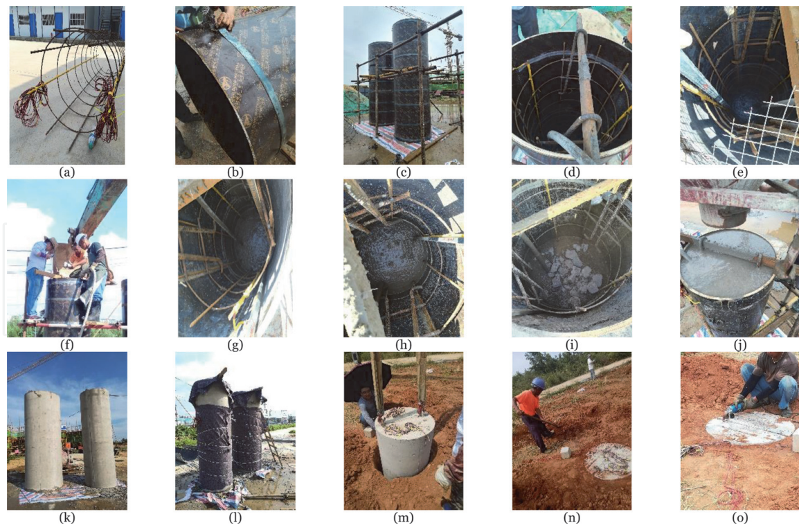
Figure 8. Construction steps of precast pier foundation filled with DCLs and fresh concrete for foundation casting. (a) Prepare reinforcement, (b) install mold, (c) set up scaffolding and molds, (d) put the steel cage into the mold, (e) cast new concrete at the bottom of the mold and then place a steel wire mesh, (f) cast new concrete incorporated with concrete lumps to the predetermined height, (g) consolidate concrete, (h) place the second layer of wire mesh, (i) cast new concrete with concrete lumps to the predetermined height and then consolidate, (j) follow steps h and i until the mold is filled, (k) demold after 1 day of curing, (l) cure pier foundation, (m) lower pier foundation into the hole, (n) fill the gap between prefabricated pier foundation and hole with undisturbed soil, (o) saw off the lifting ring to ensure the levelness of pier top end.
