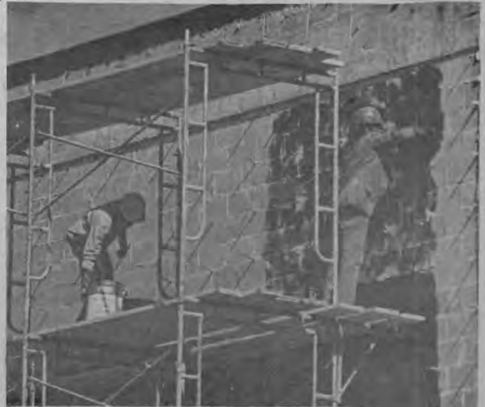
CONSTRUCTION AT THE NEW LIBERAL ARTS BUILDING— Workmen are rapidly nearing the end of construction on the new four story LA Building.
