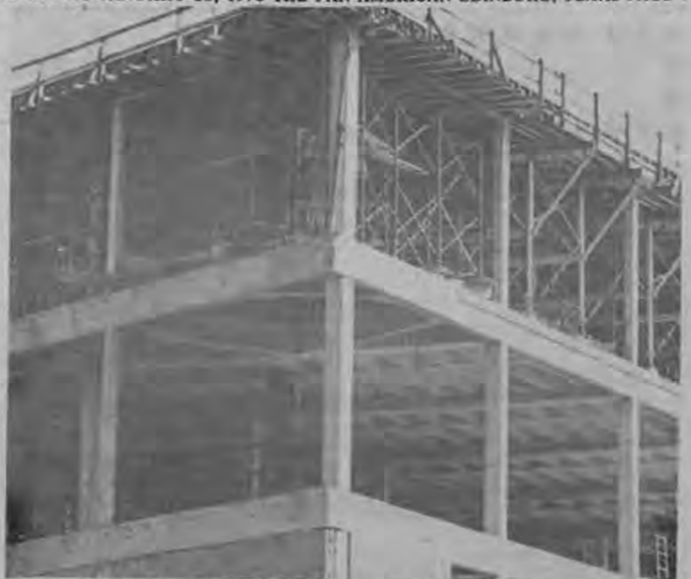
CONSTRUCTION STILL UNDERWAY AT THE LEARNING RESOURCE CENTER— The $4.5 million LRC building is still being constructed. The building which covers a total area of 141,000 square feet is set to be completed sometime in 1977.
