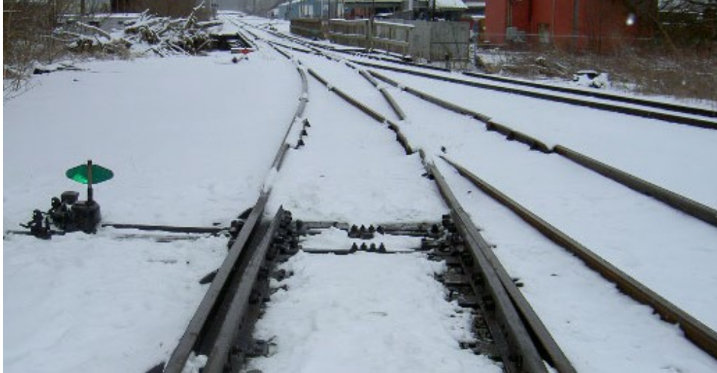
Figure 4. A track switch covered in ice and snow, creating a hazard. [25]
