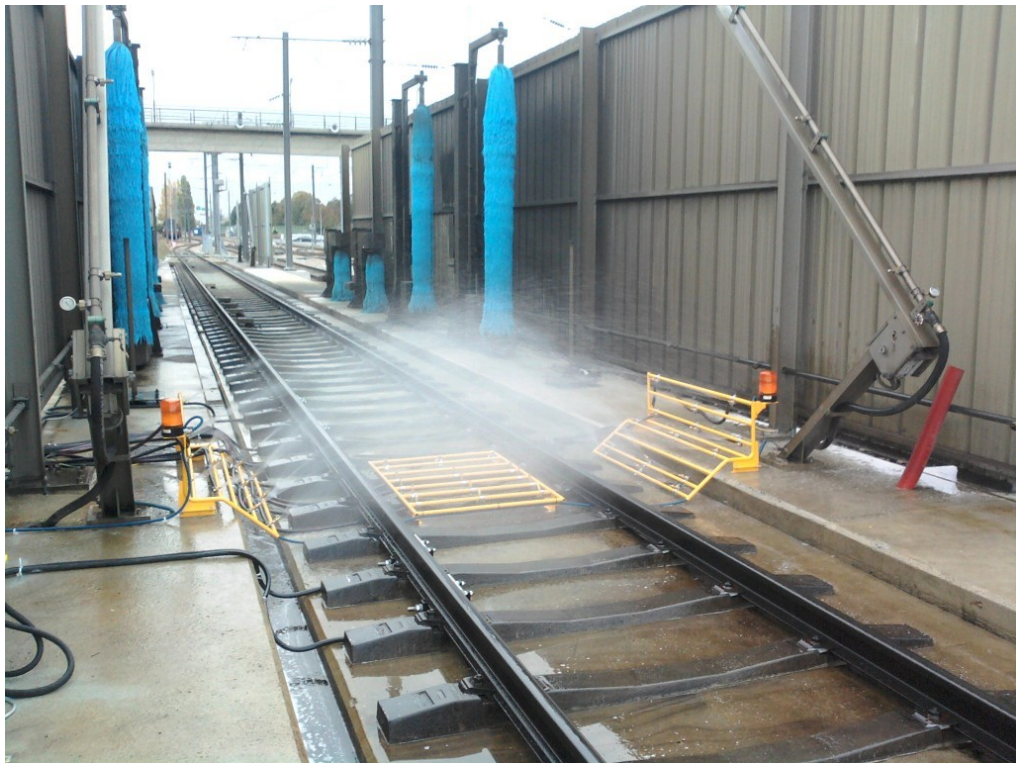
Figure 15. Train cart washing system. [77]
