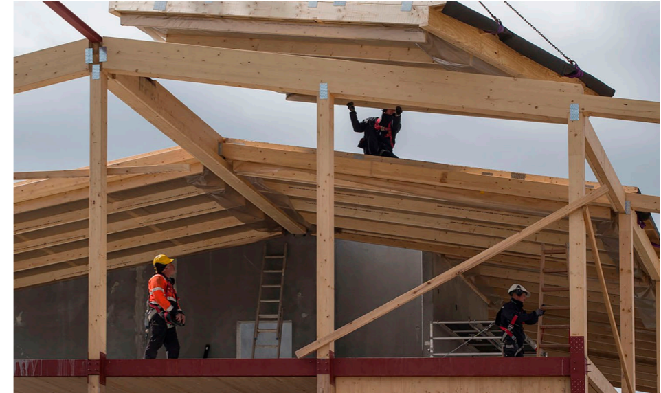
Figure 18. Gluelaminated wood posts have been connected with steel, Lisbjerg hill, Vandkunsten (Dalgaard 2019)
