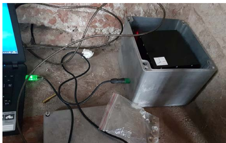
Figure 4. Sensor S.2 at level +37 m inside the tower.
