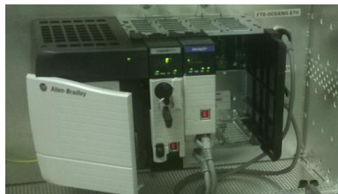
Figure 3: Allen-Bradley ControlLogix controller
