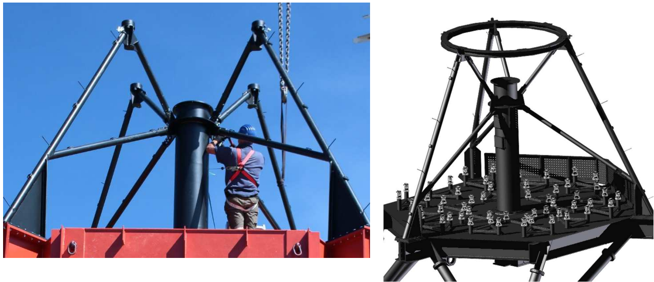
Fig 5. Prototype OSS upper structure (left) and array telescope OSS upper structure (right)
