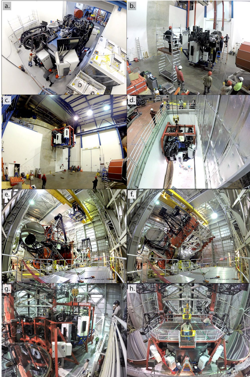
Figure 1. Final installation of LINC-NIRVANA on the LBT. The team pushes the instrument out of the mountain lab (panel a) and into the high bay, where the bridge crane assists in installing the lifting traverse (panel b). Flying the instrument from the high bay into the enclosure is an interesting challenge, since the clearance between instrument and building is only about 11mm (panels c and d). A well-choreographed “dance” with the telescope (panels e and f) allows LINC-NIRVANA to travel to the rear of the enclosure to its final mounting location (panel g). A similar dance brings the dust cover and “roof garden” into place (panel h). The entire operation took two full days.
