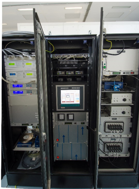
Figure 3: Thermal control cabinet (left), Instrument main cabinet (center), Calibration unit cabinet (right) were tested with all the other subsystems, satisfying the requirements.
