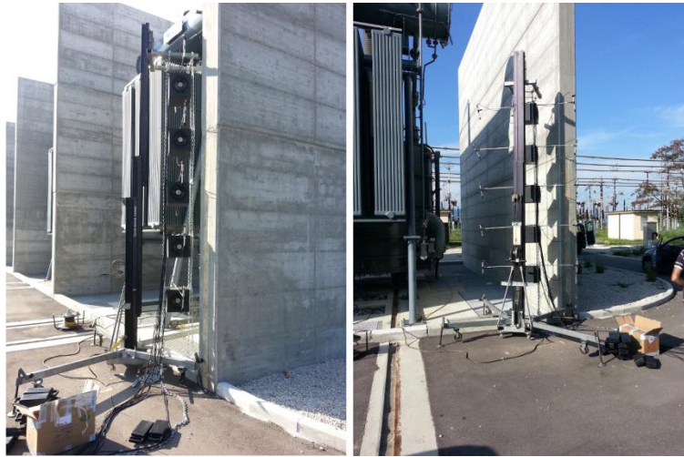
Figure 12 - Deployment of the ANC system at an electricity generation station in Tuscany (Italy).
