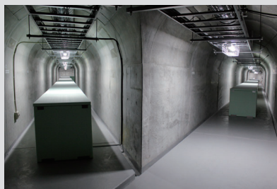
2016年に竣工した桜島の高免観測坑道 Underground tunnel to detect precursory ground deformation to eruptions, newly constructed in 2016
