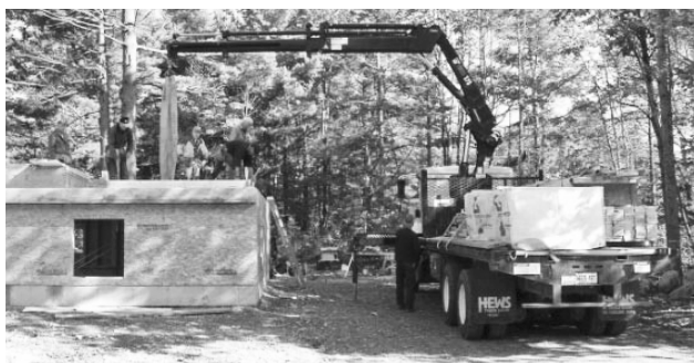
The building crew of Midcoast Habitat for Humanity at the site of its 18th house, receiving supplies.
