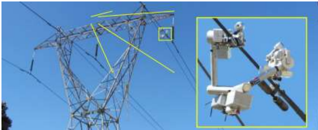
Figure 30 Power line inspection robot navigating around a damper on a 132 kV line.
