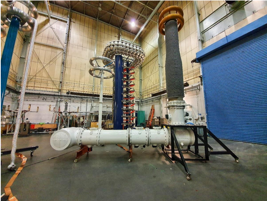
Figure 6-5. 2 MV Impulse generator test setup connected to the 420/550 kV GIB demonstrator.
