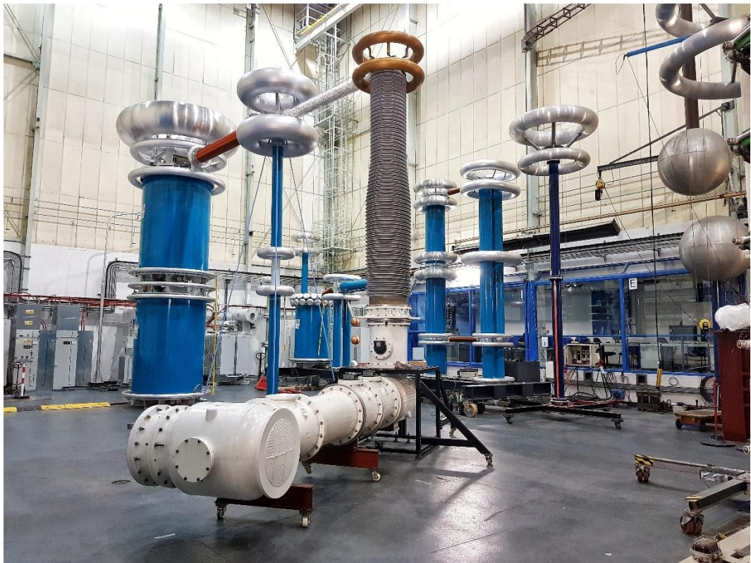
Figure 6-4. 800 kV AC generator test setup connected to the 420/550 kV GIB demonstrator.
