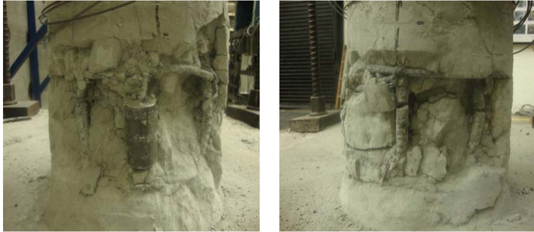
Figure 7.9 Pictures of column C1 after the test was complete.
