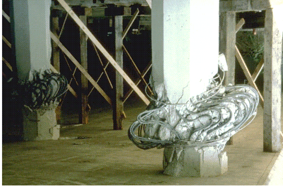
Figure 2.3 Failed RC columns under the Simi Valley Freeway as a result of the 1994 Northridge earthquake (Southern California Earthquake Data Center, 2011).
