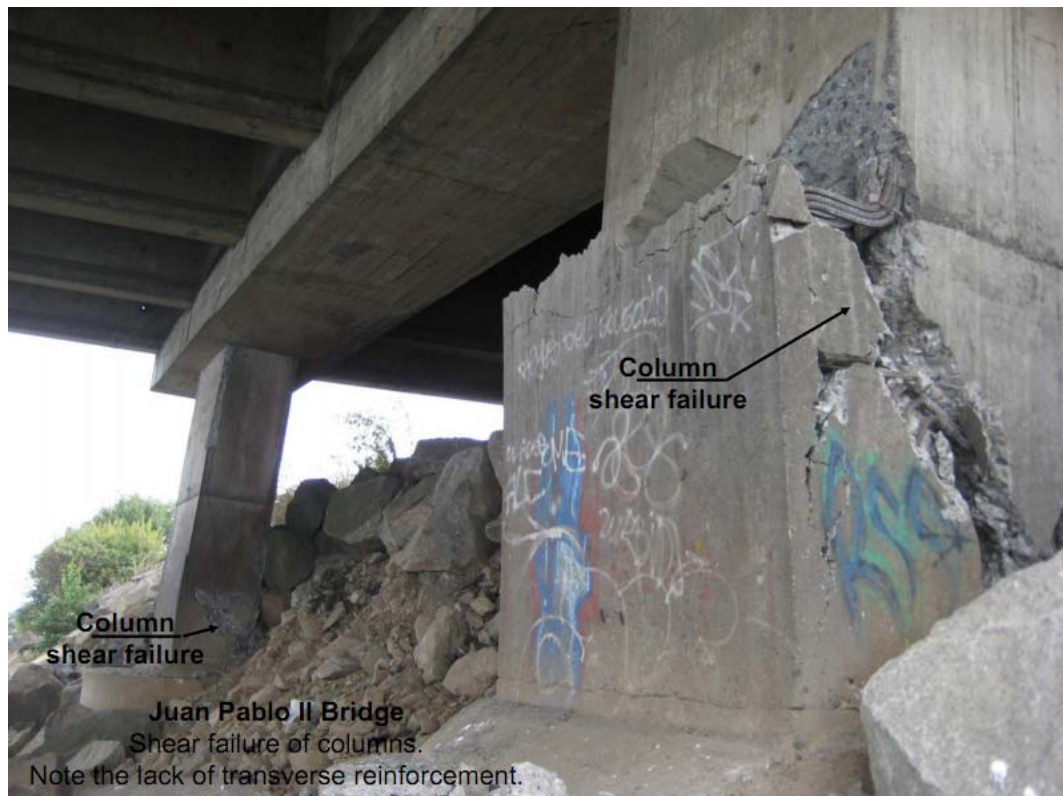
Figure 2.6 Damaged RC columns of Juan Pablo II bridge during 2010 Chile earthquake (EERI et.al, 2010).
