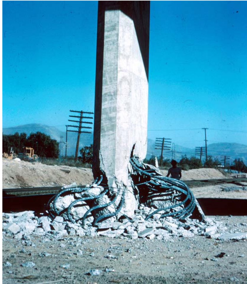
Figure 2.1 Damaged RC column on Interstates 5 and 14 during the San Fernando earthquake, 1971 (USGS, 2006a).
