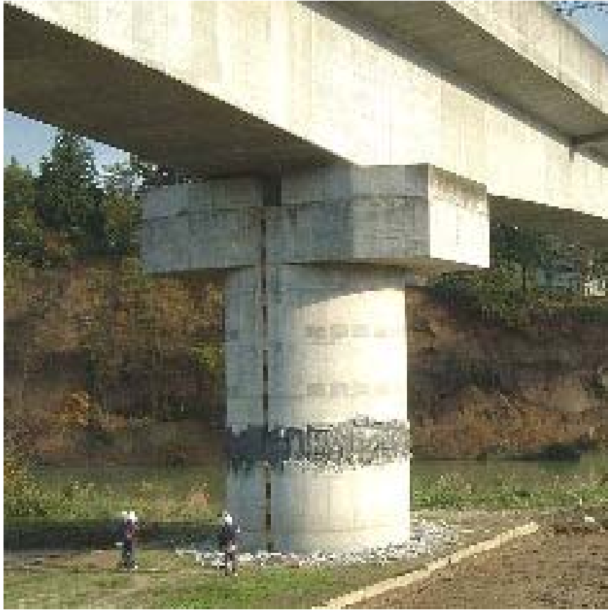
Figure 2.5 Damaged RC column of Uonogawa Bullet Train Bridge due to the 2004 Chuetsu earthquake in Japan (Shanmuganathan, 2005).
