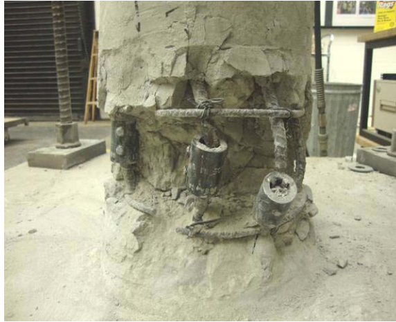
Figure 7.11 Slippage of rebars from the couplers.
