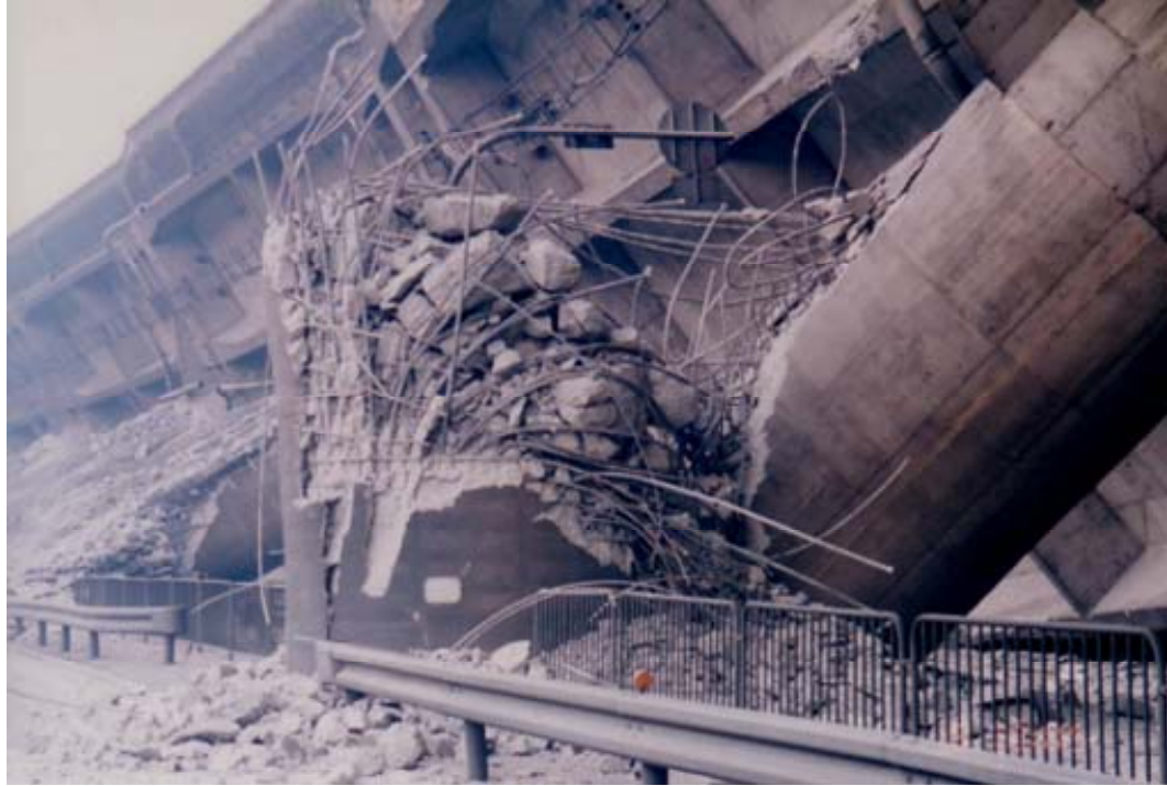
Figure 2.4 Severely damaged Hanshin expressway due to the 1995 Kobe earthquake (Kawashima, 2009)
