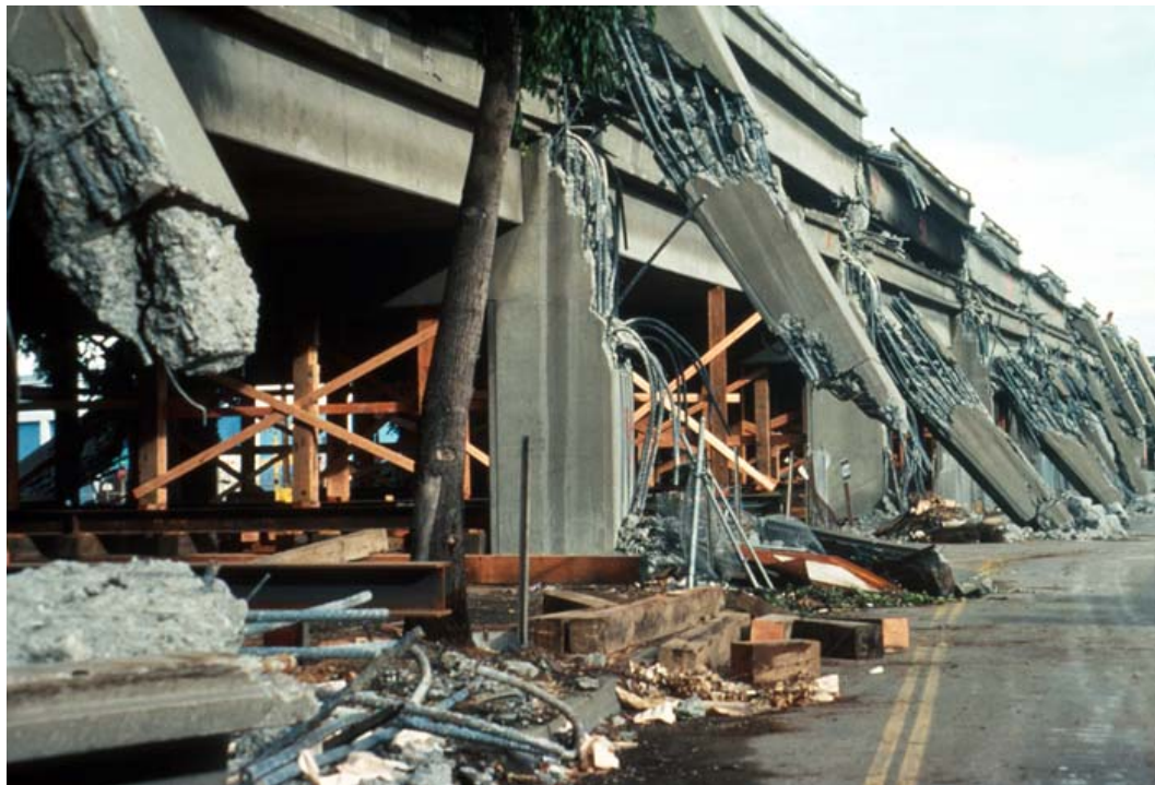
Figure 2.2 Failures of RC columns and collapsed upper deck on the Cypress viaduct of Interstate 880 (USGS, 2006b).
