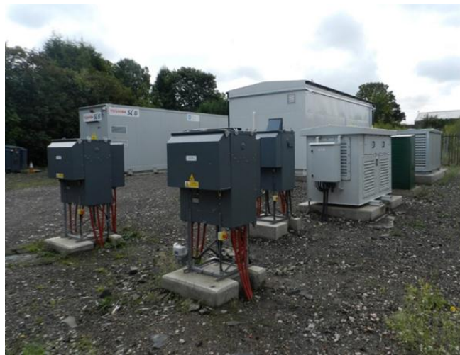
Fig. 3. Site Photo – showing battery system on the left and the inverter on the right with air handling unit
