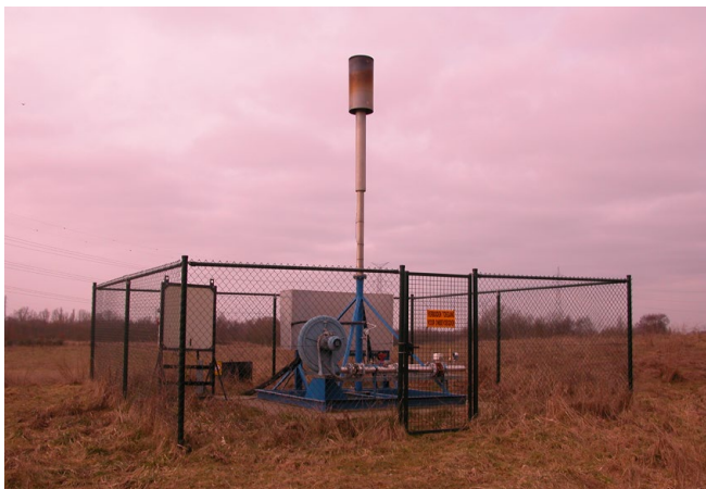
Degassing of a former landfill area, Schelle, Belgium © Public Waste Agency of Flanders
