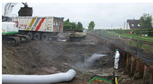
Excavation of a former waste dump, Buggenhout, Belgium © Public Waste Agency of Flanders
