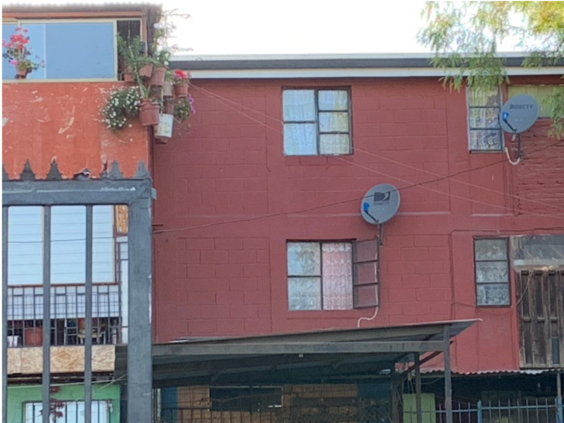
Fig. 5. Block building showing how the bricks are standing up rather than placed horizontally, evincing cheap construction and thin walls
