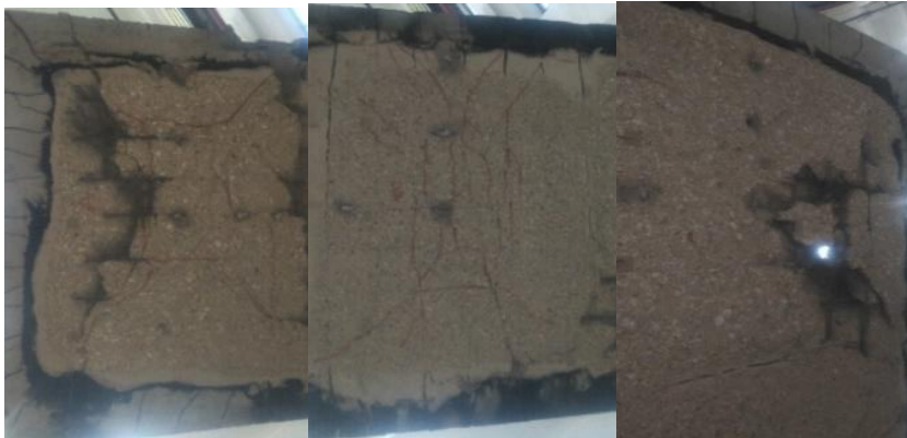
(c) Photograph of cracks on the bottom surface
