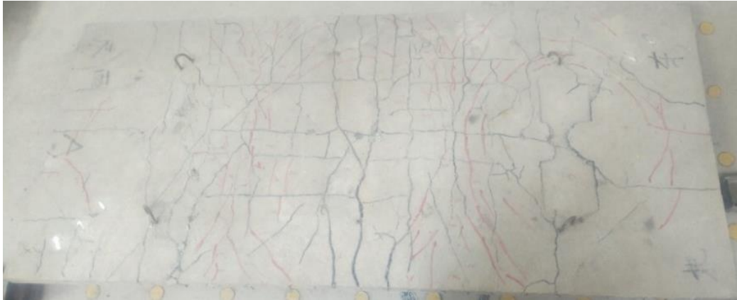
(a) Photograph of cracks on the top surface
