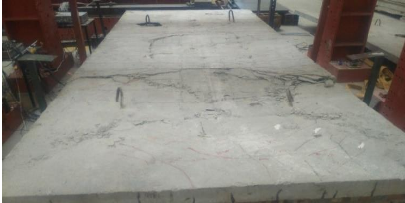
(a) Photograph of cracks on the top surface
