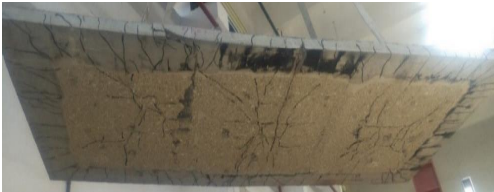
(c) Photograph of cracks on the bottom surface
