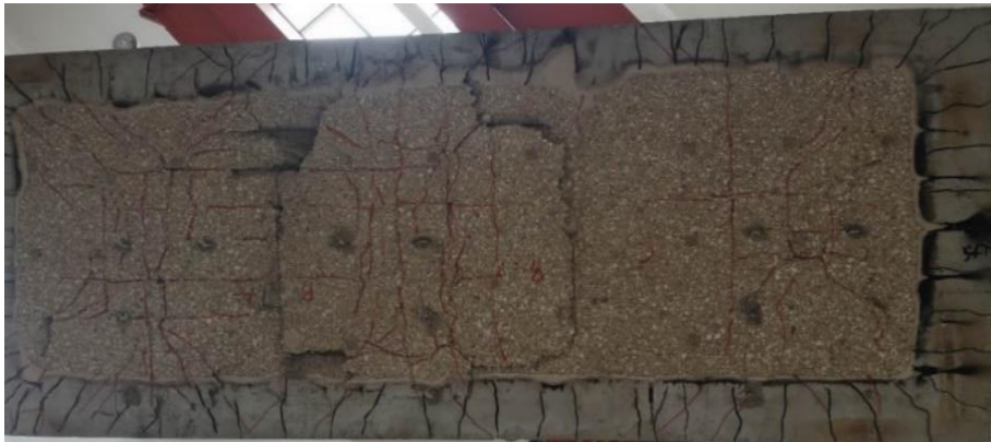
(c) Photograph of cracks on the bottom surface
