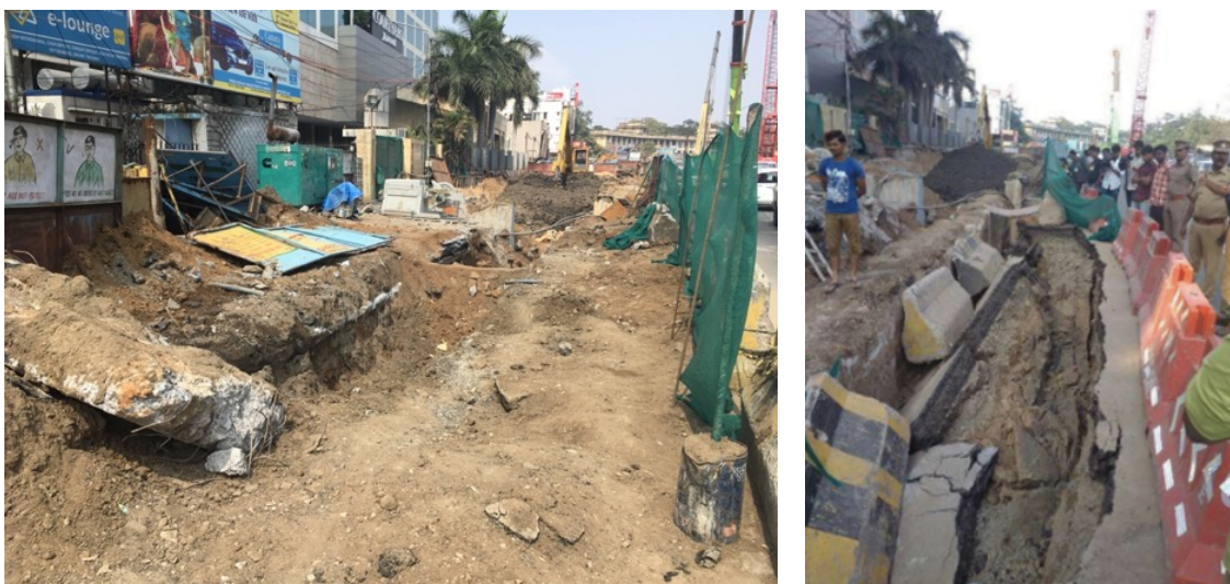
Figure 40. Collapse site, Anna Salai near DMS, January 2018. Photograph (left) by the author; (right) The News Minute.
