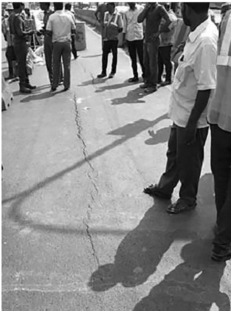
Figure 31. Cracks in Anna Salai, April 2017. The News Minute . 371
