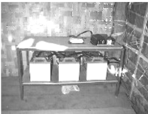
Picture 8. Installed charge controller, inverter, and batteries
