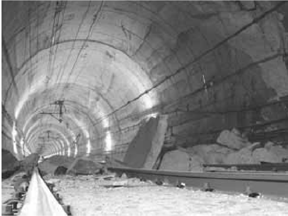
(a) Spalling of lining in Uonuma tunnel
