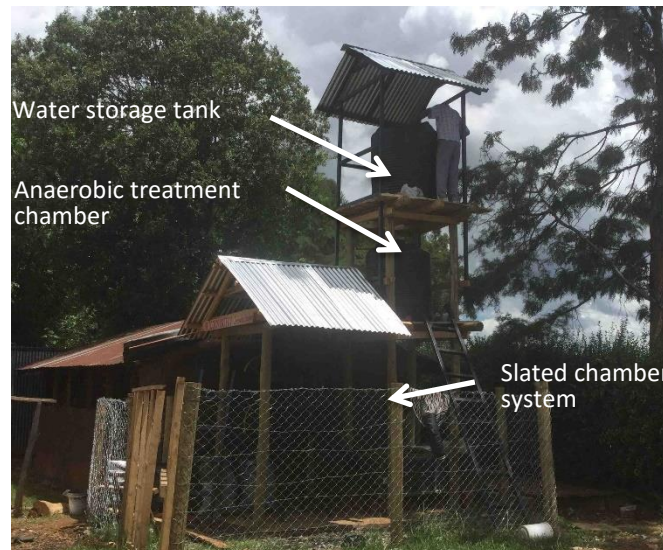
Figure 22. The on-site water recycle system in Cheplaskai secondary school
