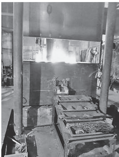
Figure 1 Ore-thermal furnace RPZ-300 kVA
