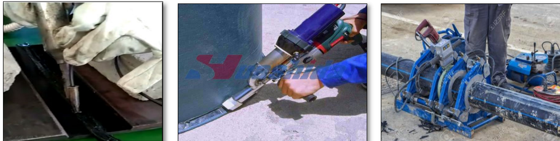
(a) (b) (c) Gambar 3.(a). Hot gas welding (b) Butt Fusion Welding (c) Butt Fusion Welding
