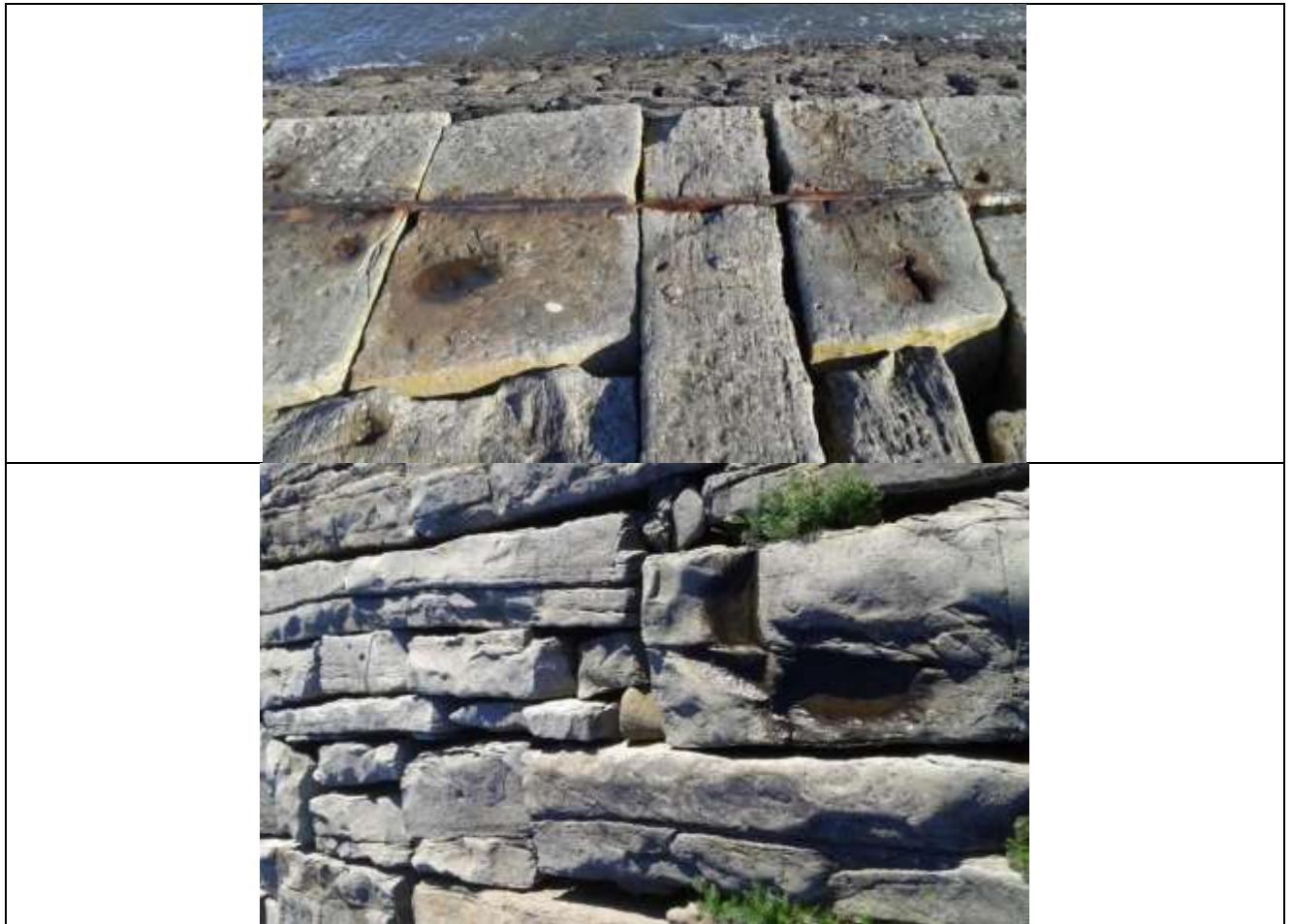
Figure D.3 Granton East Breakwater details, a) edge rail; b) end-on blockwork, 2017
