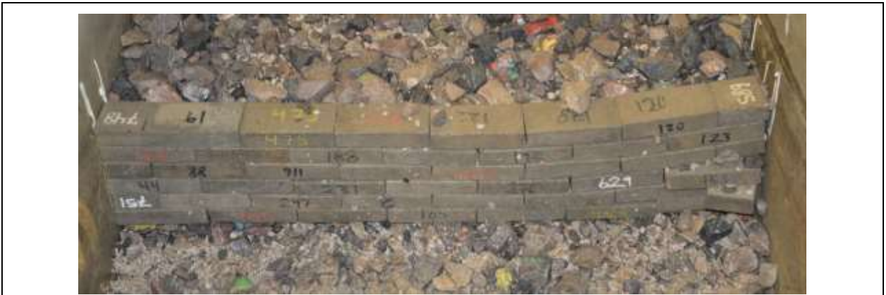
Figure 7.16 Excavated front wall, note vertical arching where foundation has scoured
