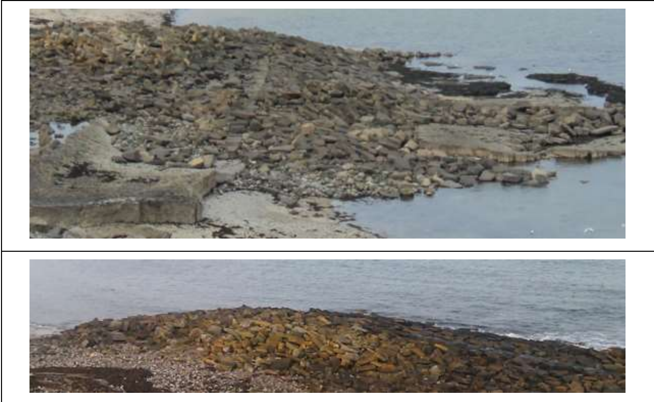
Figure 2.30 Collapsed breakwater at Skateraw (2014)
