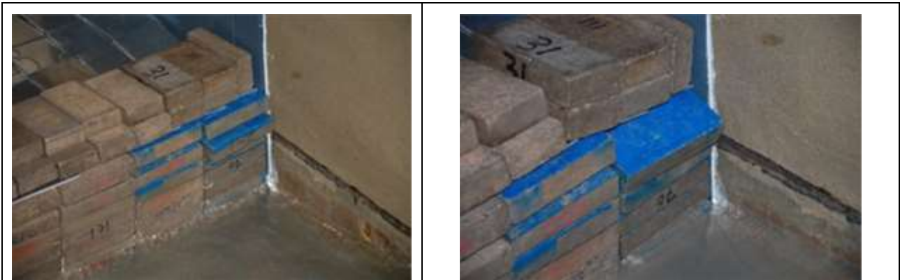
Figure 7.28 Onset of damage during Tests 138 and 139
