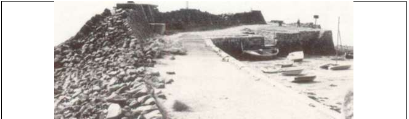
Figure D.7 Pettycur breakwater, damaged crown wall
