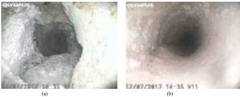
Fig. 8. Videoendoscopy V11 – from intrados: (a) View at 15 cm from the start of the drill, filling in unbound material; (b) Image at 5 cm from the start of the drill, brick and mortar elements.
