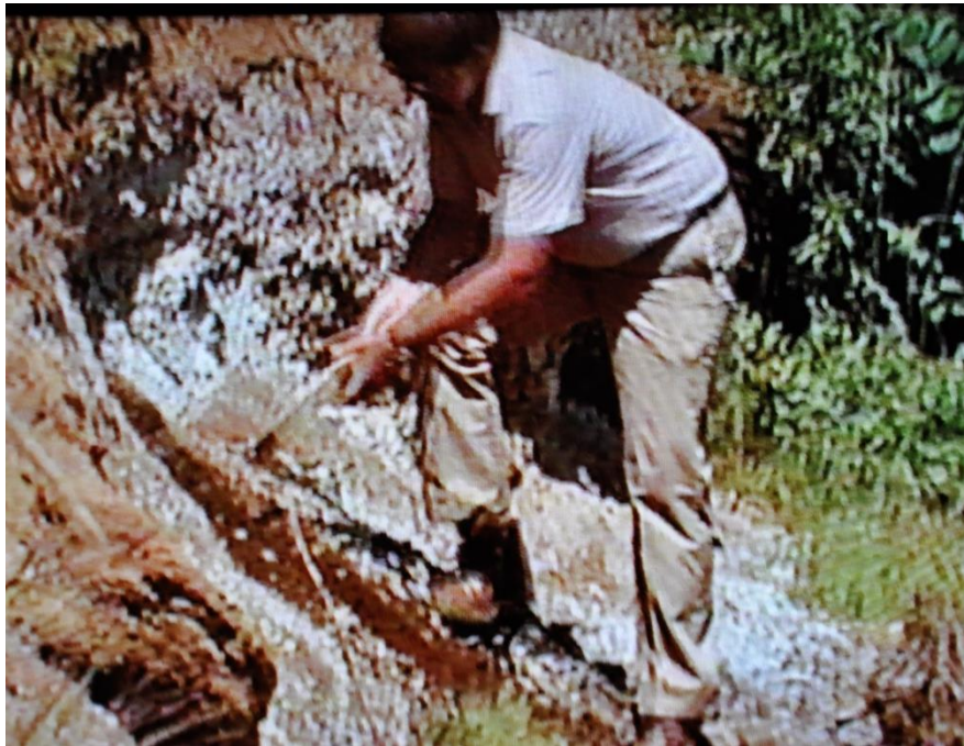
Figure 5.5. Water-soluble efflorescent salts (Cottonwood Productions, 1986).
