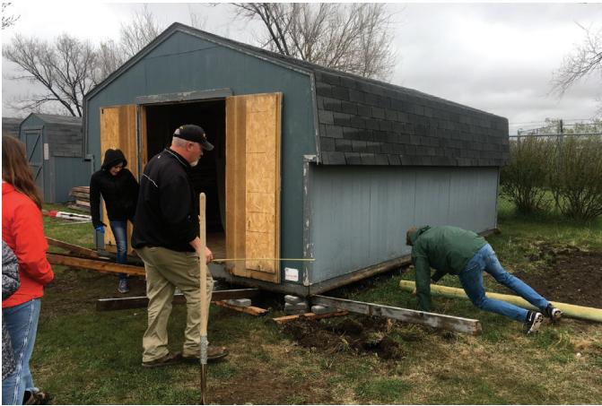
Figure 2. Team members moving a shed to prepare the area for greenhouse construction.
