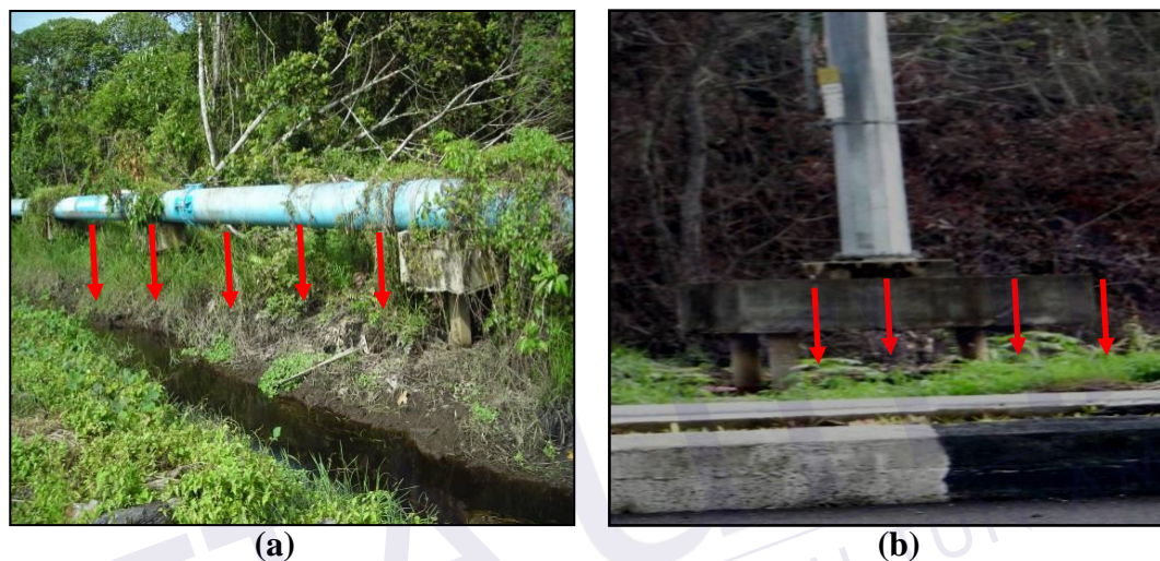
Figure 1.3: Settlement for (a) pipeline and (b) lamp post near Salim-Airport Road By-Pass, Sibul, Sarawak (Author, 2009)
