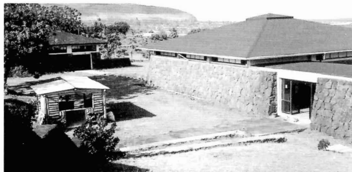
A coffee house is under construction near the entrance to the Sebastián Englert Museum.
