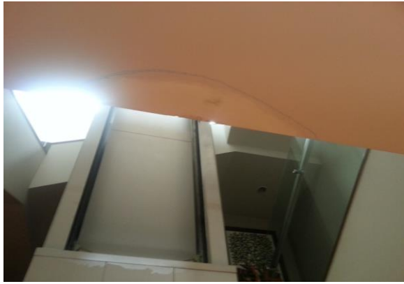
Fig. 1. Picture is showing the offending margin of roof of the corridor.
