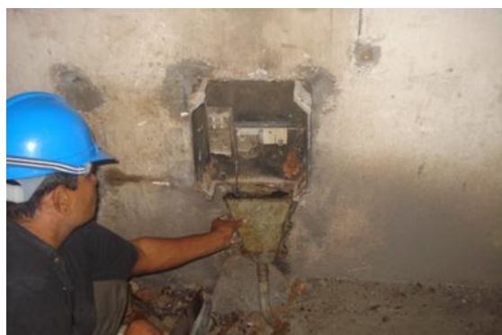
Fig. 4. The electric appliance fixed to the wall was severely burnt and exploded.
