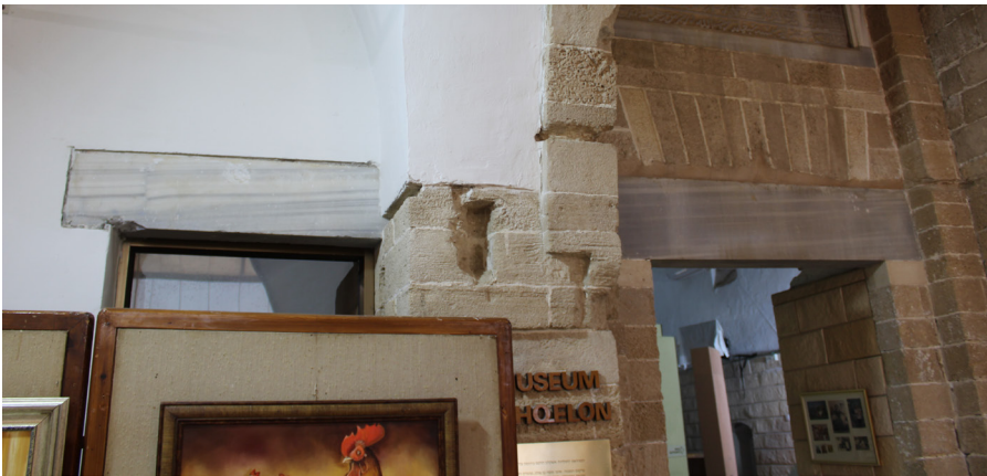
fig. 17a-c. Architectural artifacts reused in the mosque in Majdal, Ashkelon (photo author 2019).
