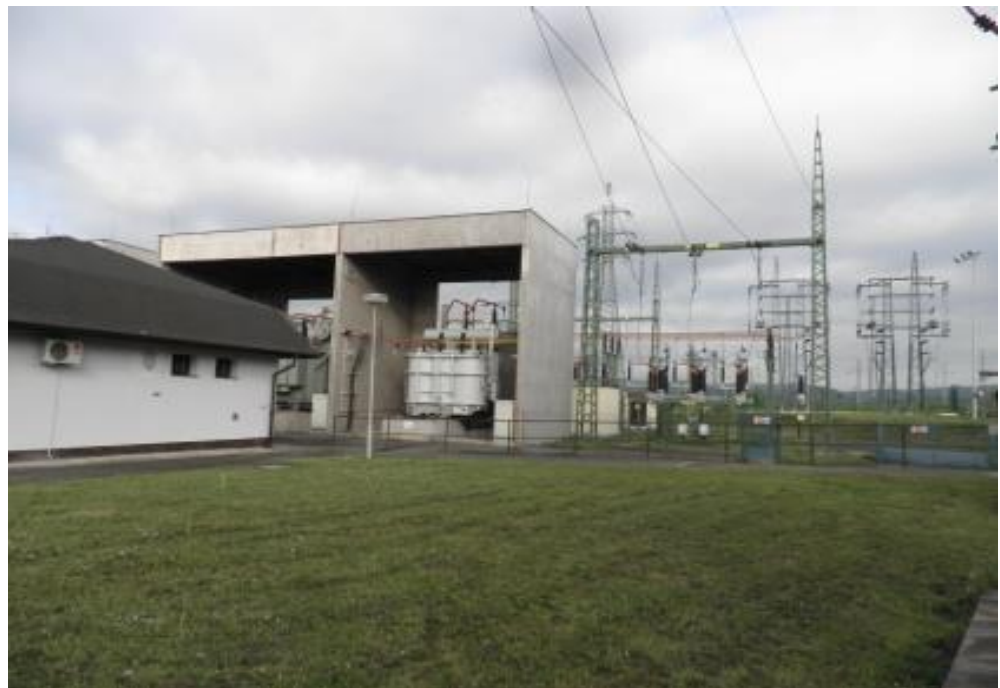
Figure 3. View of traction substation 25 kV/50 Hz.
