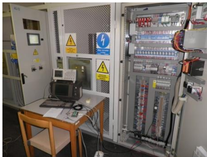
Figure 13. View of the measuring stand at the traction substation.
