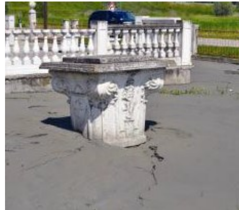
d) bearing capacity failure
