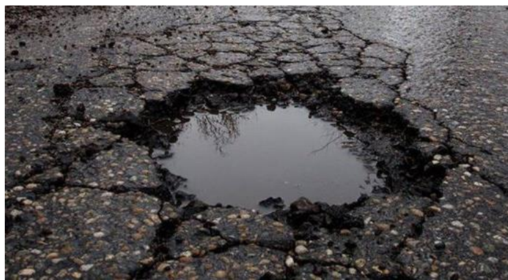
Figure 1. Pothole on the road.
