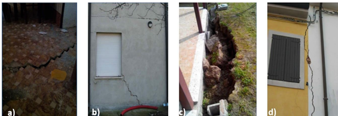
Figure 6-39 Examples of the most typical liquefaction-induced building damage in the municipality of Terre del Reno.
