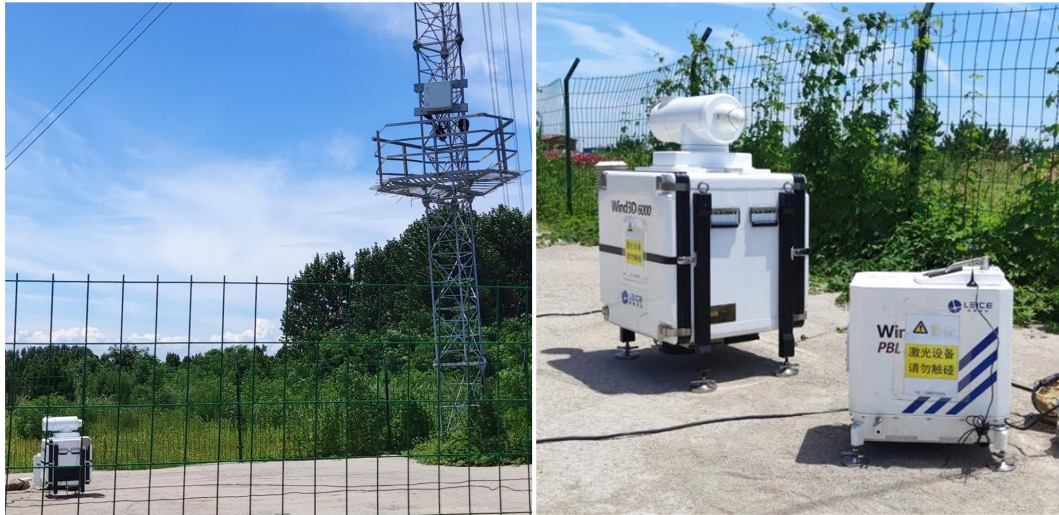
Figure 2. Photos of the CDLs and the mast onto which the cup anemometers and the wind vines were mounted at the Haiyang site.
