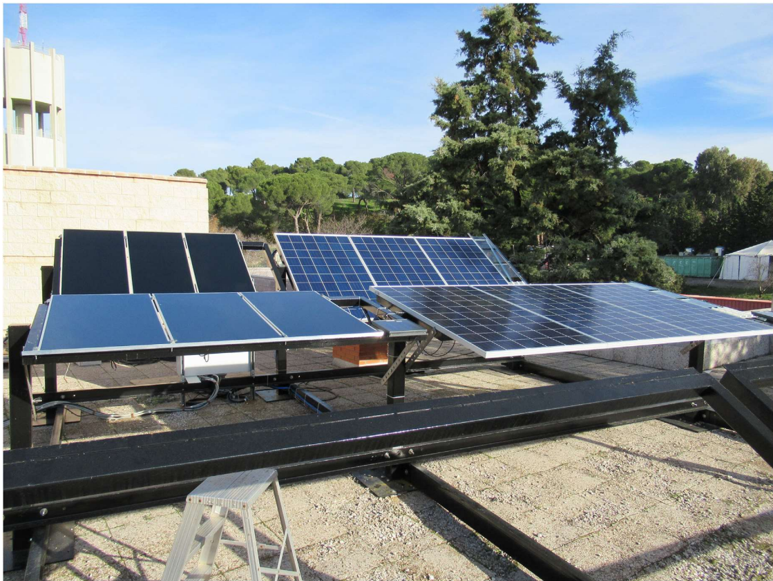
Fig. 1. Picture of the PVCastSOIL facility in the rooftop of one building at CIEMAT.
