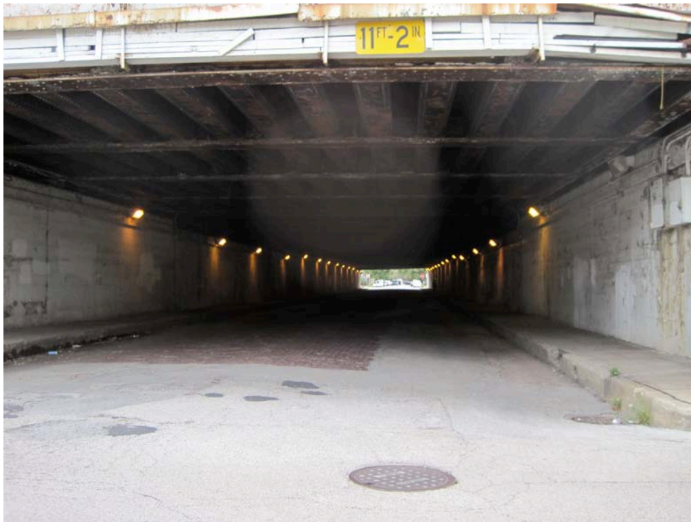
Figure 19: The channel under the railroad viaduct at the west side of the Chinatown connecting the community to the West Side ghetto. It was deemed dangerous to cross through the channel which has a
