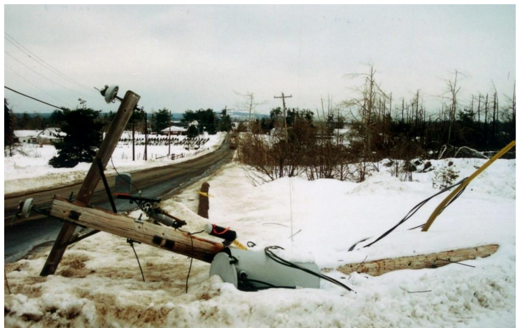
Figure 2. Example of icing impact on a medium voltage distribution line (1998 Eastern Canada ice storm, credit: private archive).
