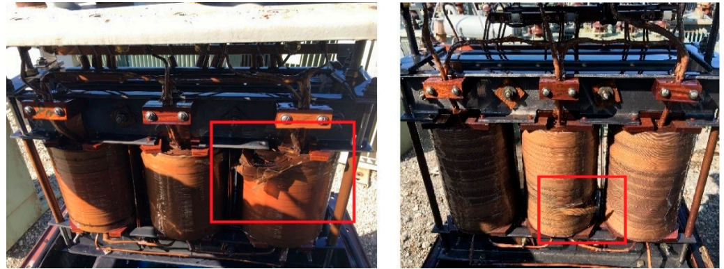
Figure 1. Deteriorated solid insulation of distribution transformers.
