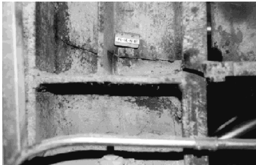
Figure 1-1 Fractured connection in a steel moment frame
