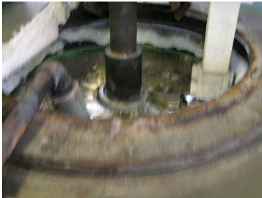
Figure 4-22: Immersion of the Roll and Scraper Assembly (End)
