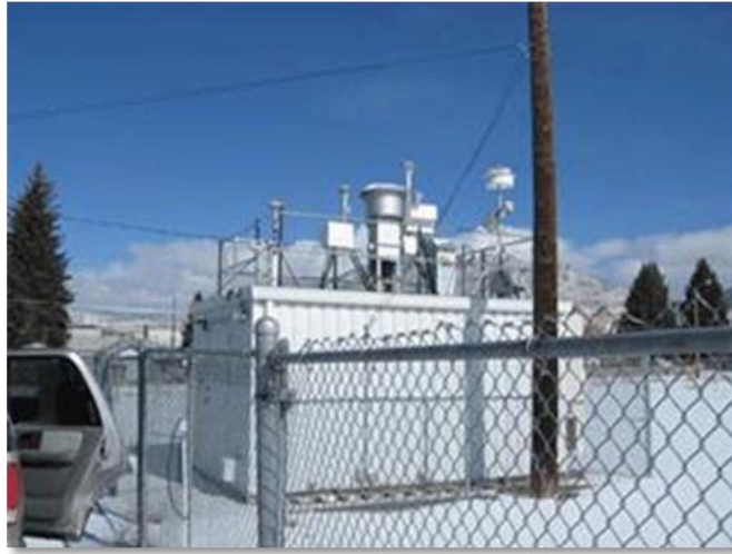
Figure 1: Greeley School Monitoring Station
