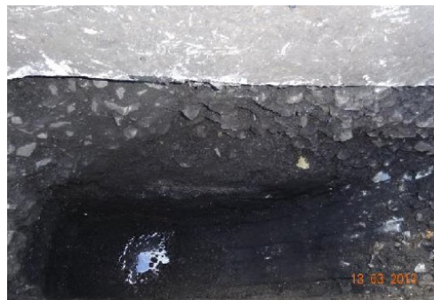
Fig. 7 Ballast highly fouled by fines and perched water in ash
