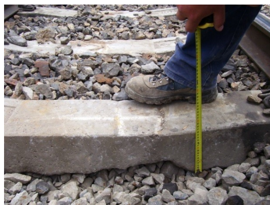
Fig. 3: Centre-bound-type failure (directly caused by poor ballast condition)
