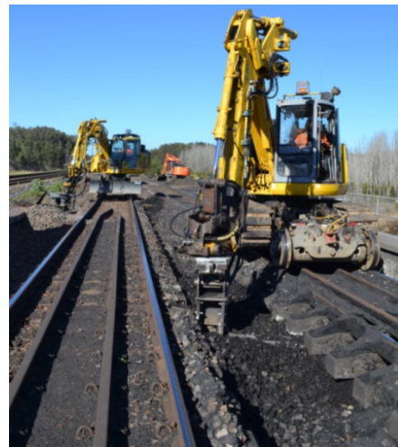
Fig. 11 Hi-rail based undercutting machine is carrying out the track bed undercutting work
