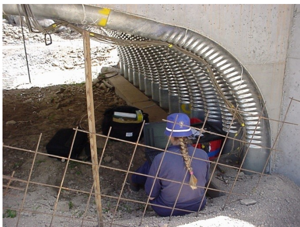
Fig. 3: A long span deep-corrugated reinforced steel box culvert under testing by Ingal Civil Products, Queensland, Australia, 2002.
