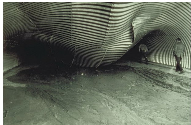
Fig. 2: Collapsed roof of a steel culvert structure, USA, 1979.
