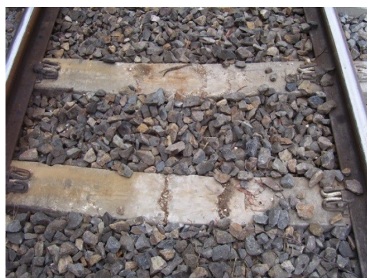
Fig. 2: Severe worn at the base of middle section (usually combined with center-bound-type cracks on the top surface of middle section)
