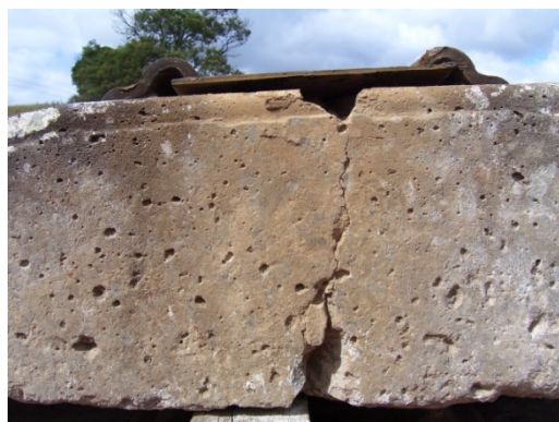
Fig. 1: Bending crack at the rail seat area (cracks initiating underneath the concrete sleeper and extending through the whole cross section of the sleeper to the rail seat)
