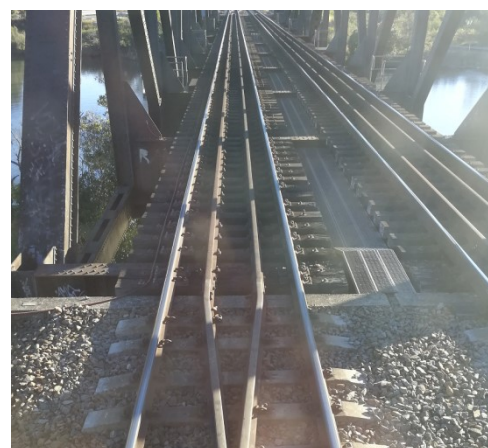
Fig. 5 Delkor ALT1 pads are needed to be installed on the ballast logs of the steel girder bridges
