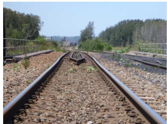
Fig. 4 Track shows dip in track at bridge transition.
