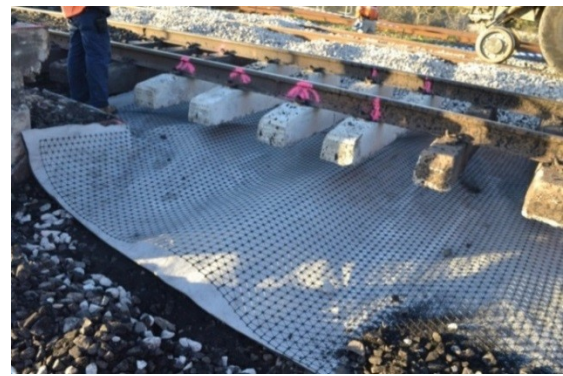
Fig. 14 Tracktex combined with Tensor SS40 geofabric at the concrete bridge transition area
